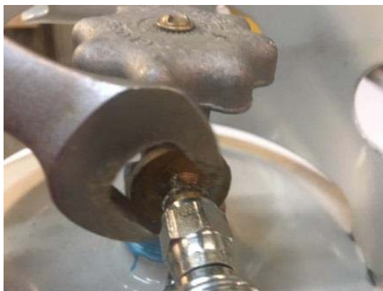
Hose to cylinder connection
